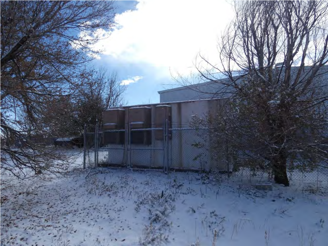
Nextel Equipment Shelter
