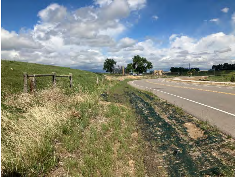
(Left) Road side swale along toe of dam and adjacent to N. 111 th Street. Riprap will be installed in swale and toe drain installed in vicinity of fence
