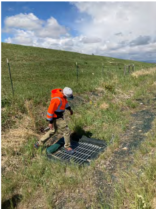
(Above) Storm sewer inlet located along road side swale. Toe drain will connect into storm system at this location.
