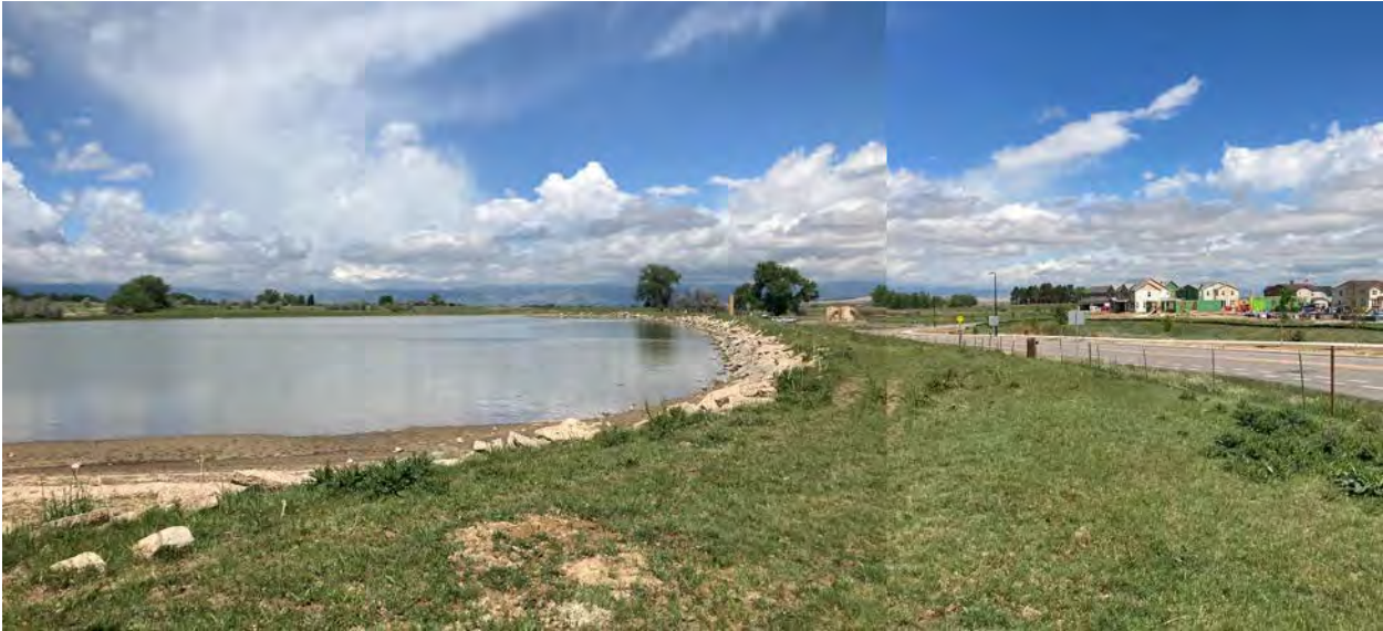
Prince Lake No. 1 dam embankment taken from spillway way looking along N. 111 th Street. Embankment height to be increased by 1 foot and rubble embankment material to be replaced with standard riprap.
