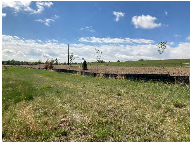
(Above) Bottom of recently-constructed drainage channel adjacent to N.111 th St. PPDam embankment seen in background. Bare earth above silt fence is the planned location for the Turf Reinforcement Mat.
