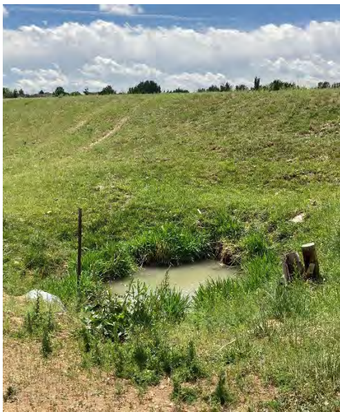
(Above) Downstream end of current outlet pipe to be replaced.
