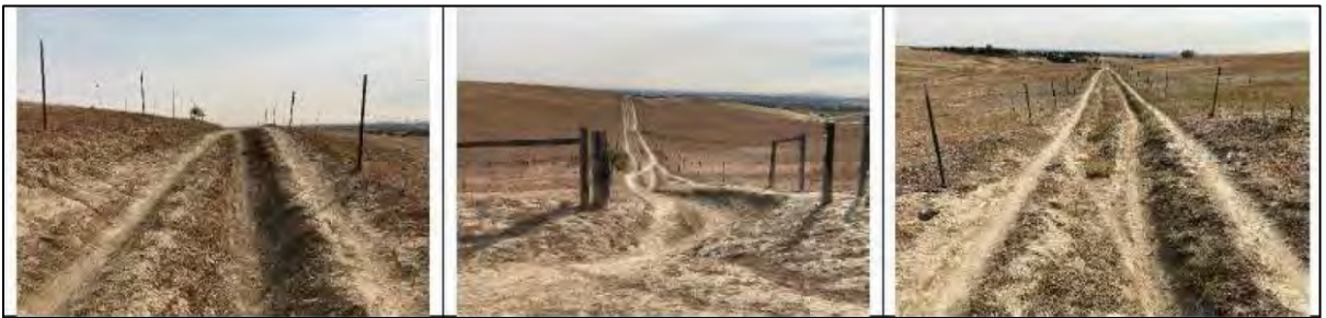
Figure 3: Erosion on existing trails to be repaired
