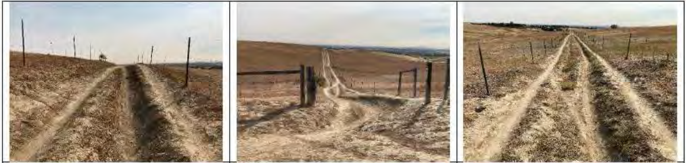
Photos 3-5. Erosion on existing East Boulder Trail to be repaired.
