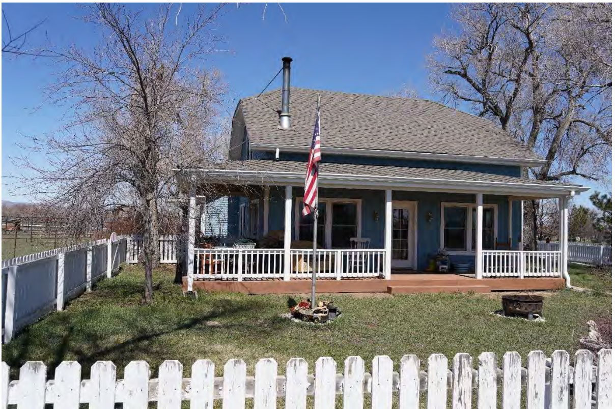
Figure 10: Southern façade of the residence with unpermitted porch addition, staff photo taken April 6, 2023
