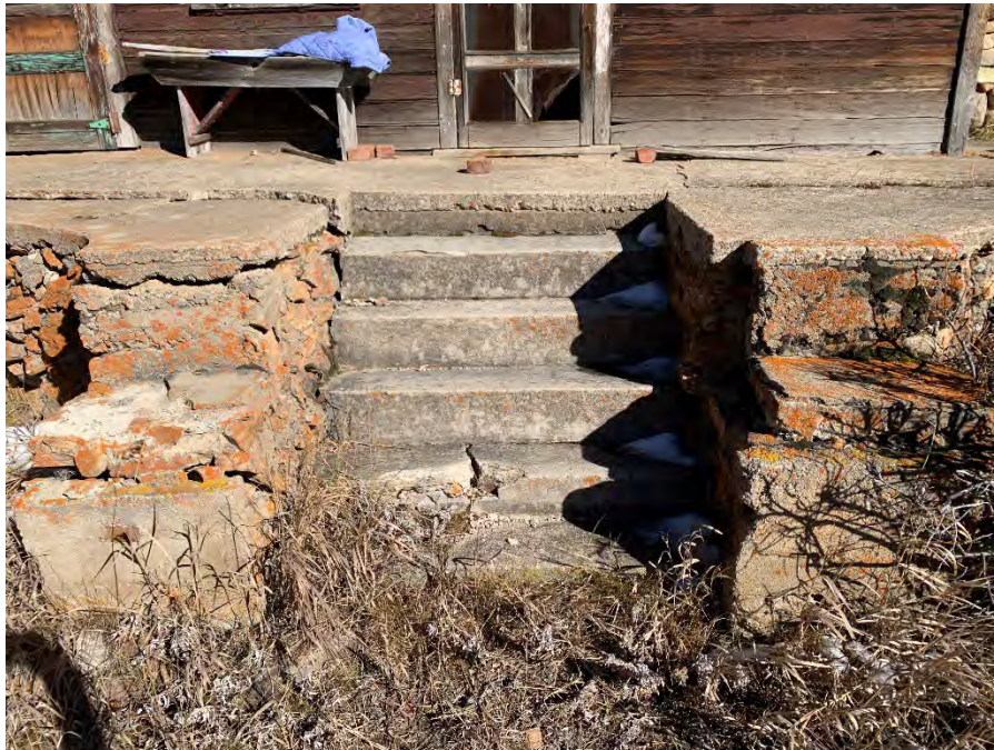
Figure 8: Stairs up to the concrete patio along the west side of the cabin.
