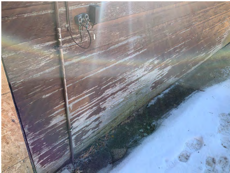
Figure 35: Deterioration typical at the lower section of the exterior walls
