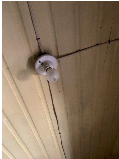
Figure 103: Light fixture located in the kitchen.
