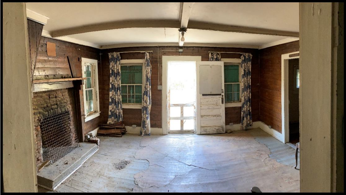
Tucker Cabin – living room overview after interior cleanup and before interior temp wall installed
