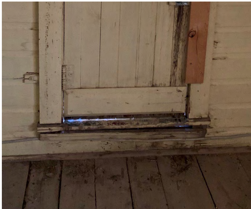
Figure 79: Water damage below the threshold at the second floor door opening.
