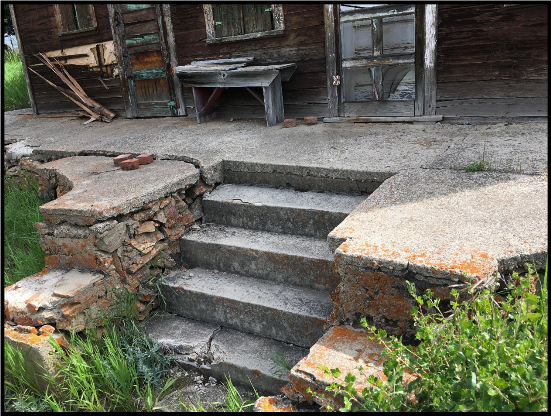
Tucker Cabin – exterior concrete porch detail showing damage with cabin siding damage in background
