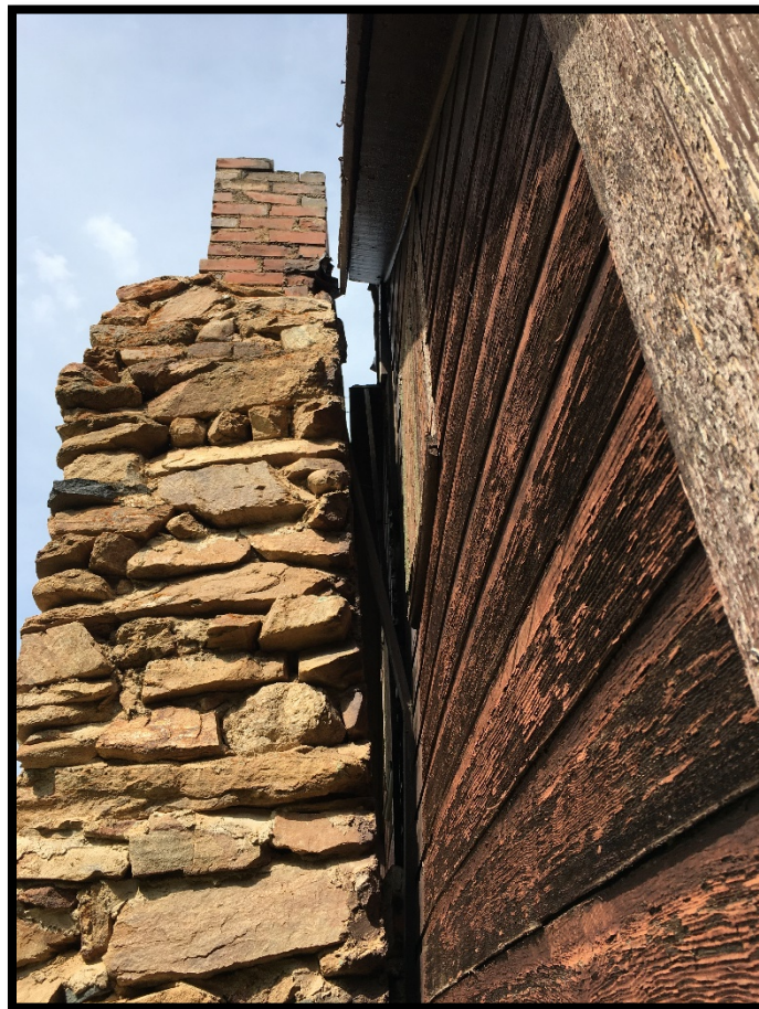
Tucker Cabin – exterior stone chimney detail showing large separation away from building exterior
