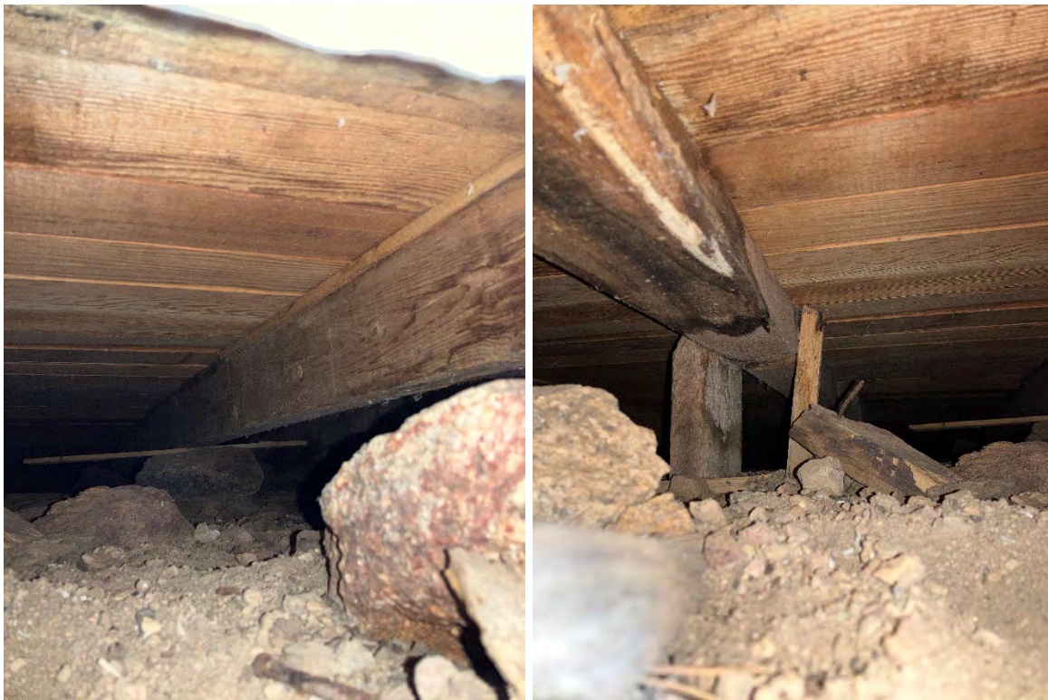
Figure 26: Examples of first floor framing as seen from a small opening on the west elevation. Note the sporadically placed stone and wood props, and the water staining visible on some of the joists.
