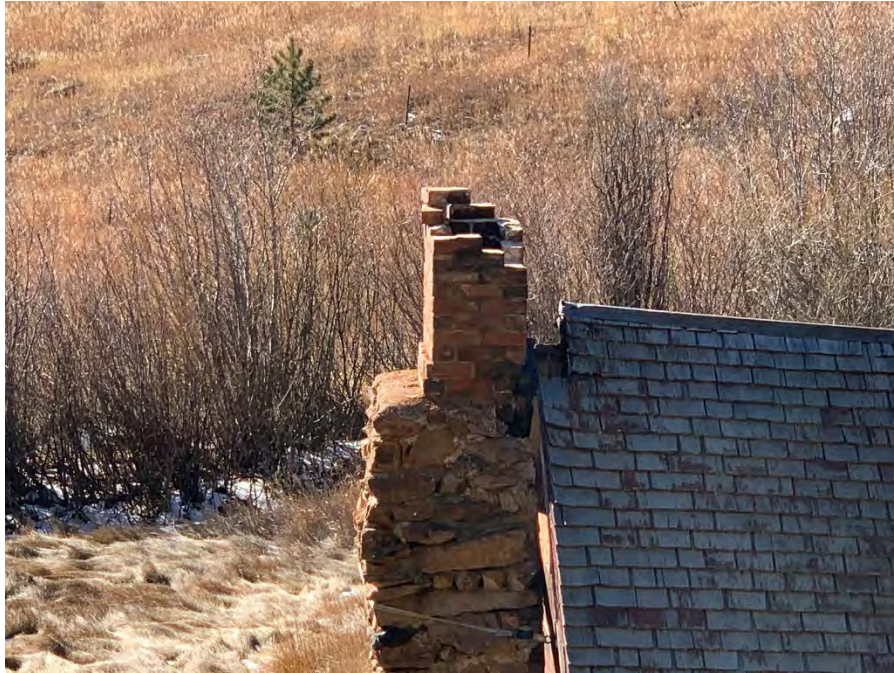
Figure 45: Detail view of roof condition adjacent to the south chimney.
