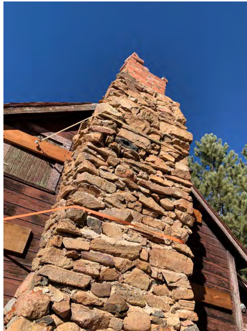
Figure 37: Upper section of the stone chimney on the south elevation of the cabin.
