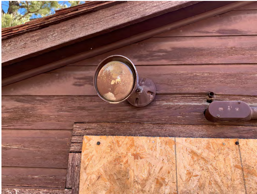
Figure 101: Modern single lamp light fixture located at the east end of the north elevation.
