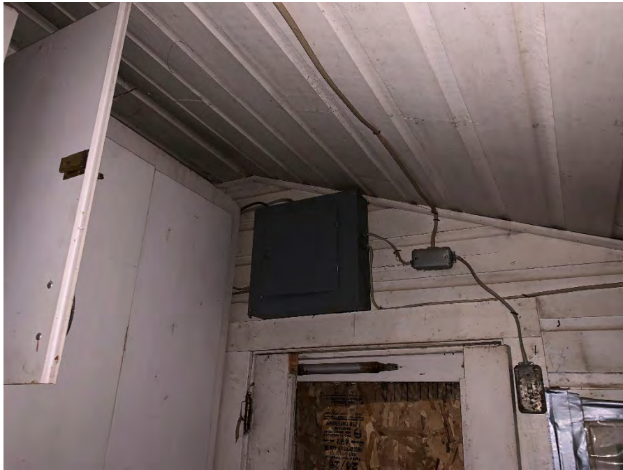
Figure 99: Electrical panel and distribution on the north wall of the kitchen.
