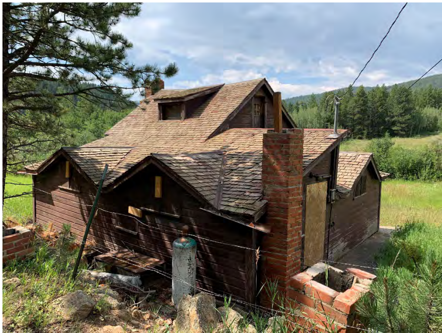
Figure 44: Roof from the northeast corner of the building. Note area of damage on the gable dormer and ridge cap due to the chimney failure.
