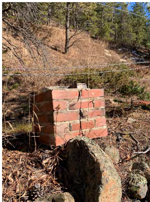
Figure 40: Upper section of the brick chimney to the northeast of the building.
