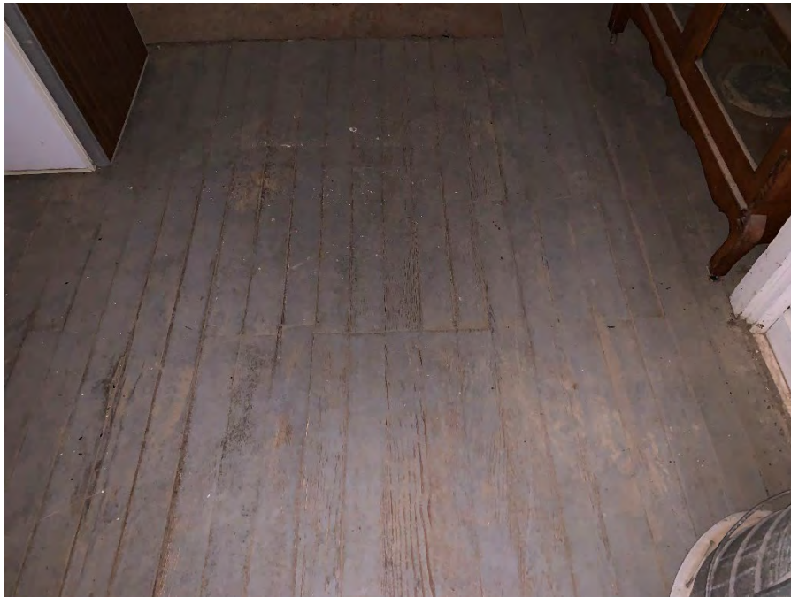
Figure 87: Joint noted in kitchen flooring.
