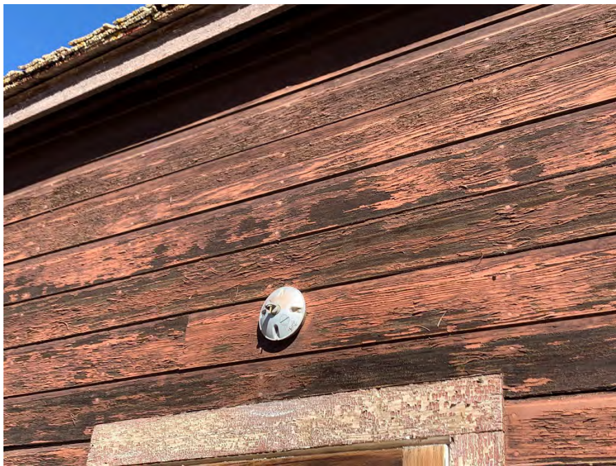
Figure 100: Light fixture location above the living room entrance on the west elevation.
