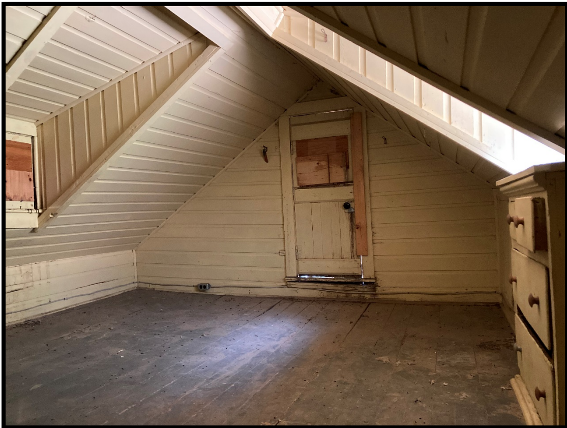
Tucker Cabin – 2 nd floor bedroom with sagging unsafe floor after interior cleanup
