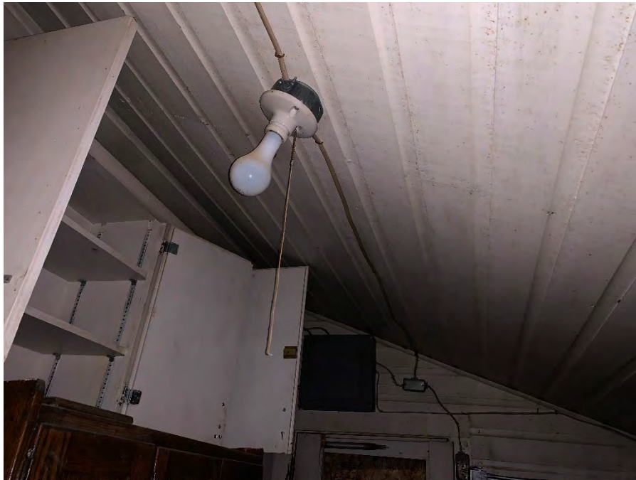
Figure 104: Light fixture located in the kitchen.
