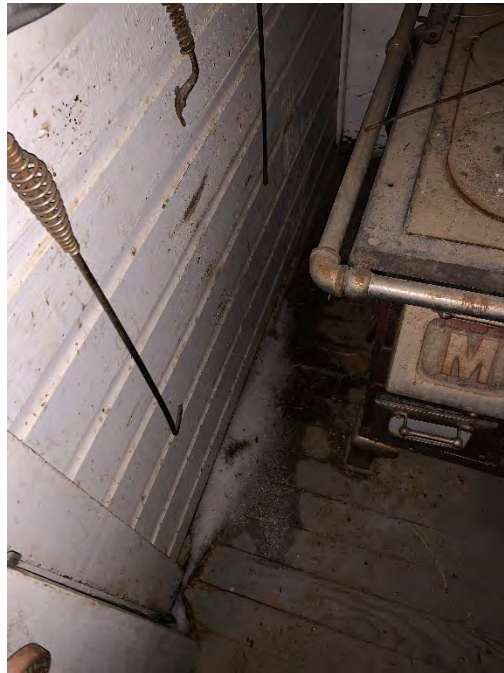
Figure 86: Snow observed in the kitchen.
