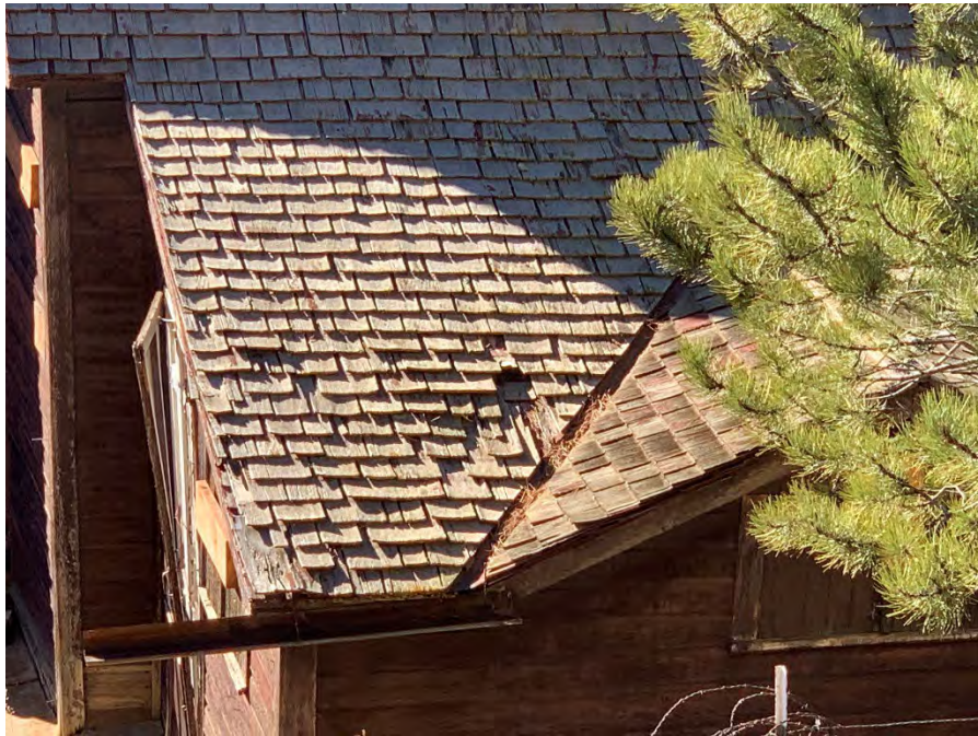
Figure 43: Detail view of missing shingles on the east slope of the roof.
