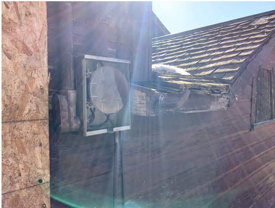
Figure 98: Electrical service equipment on the north elevation.
