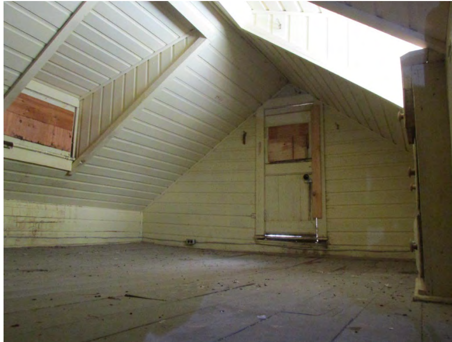
Figure 28: Second floor. Note there are no collar or rafter ties at the main gable roof
