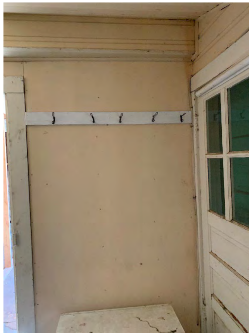
Figure 77: Gypsum board wall finish on the south wall of the first floor bedroom.
