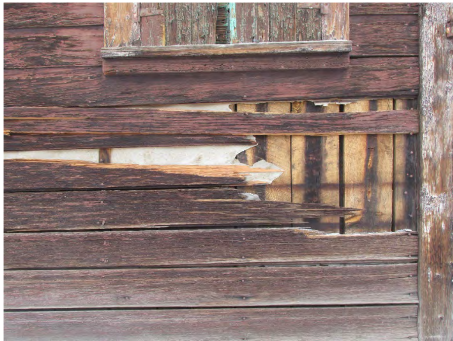
Figure 29: Exterior wall, area of missing siding. Note 2 layers of 1x sheathing.
