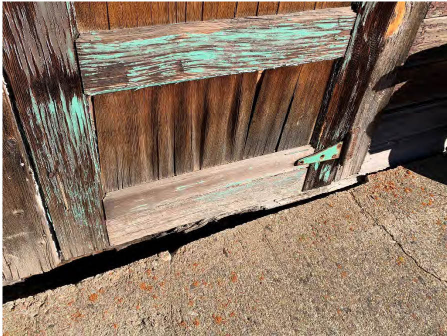
Figure 20: Gap at door threshold on the west elevation.
