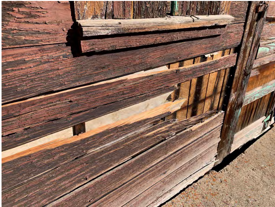
Figure 32: Painted wood siding on the west elevation. Note area of damage will require replacement.
