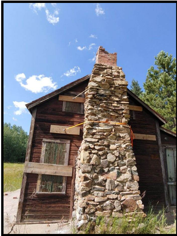
Tucker Cabin – exterior stone chimney with emergency strapping in place to prevent chimney failure
