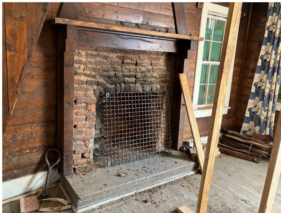
Figure 31: Brick fireplace of the south chimney, note arch-shaped cracks above shallow arch
