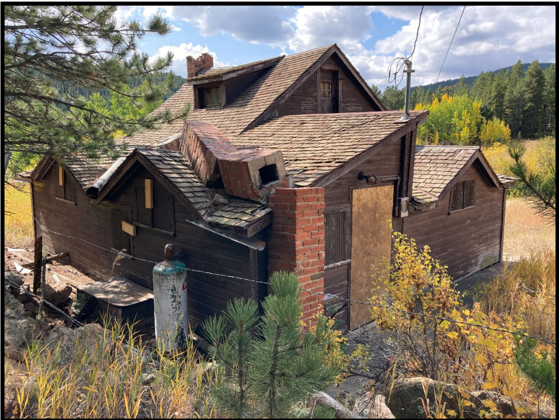
Tucker Cabin – northwest elevation showing collapsed red brick chimney on roof
