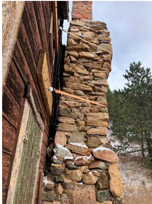
Figure 30: Stone chimney strapped to south elevation of the cabin. Note gap between cabin and chimney widens along the height indicating outward lean.
