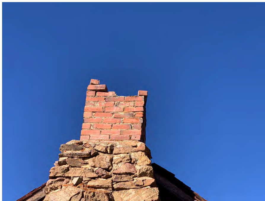
Figure 38: Detail view of brick condition at the top of the south elevation chimney.
