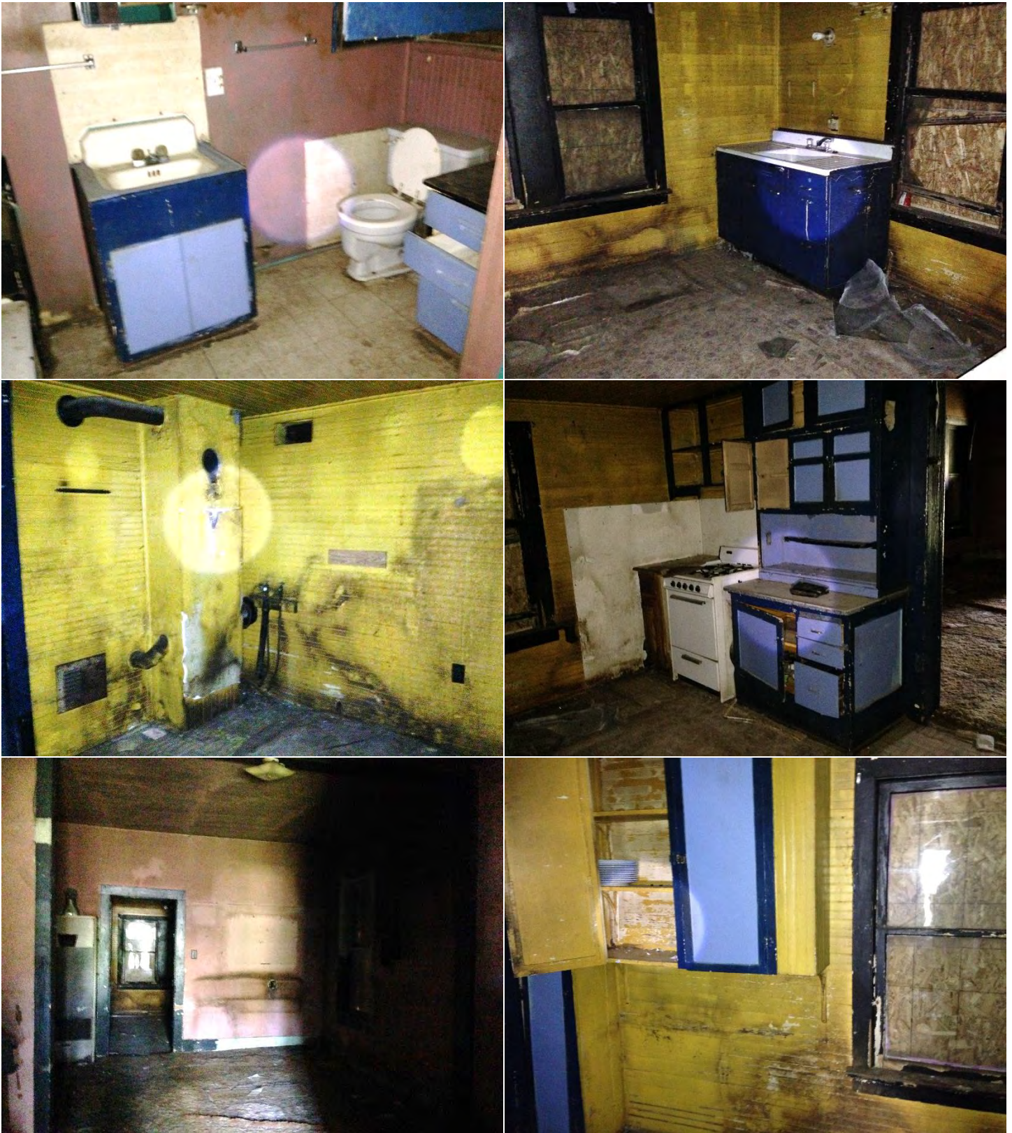
Some photos of the house interior. The floor was covered with rat feces.
