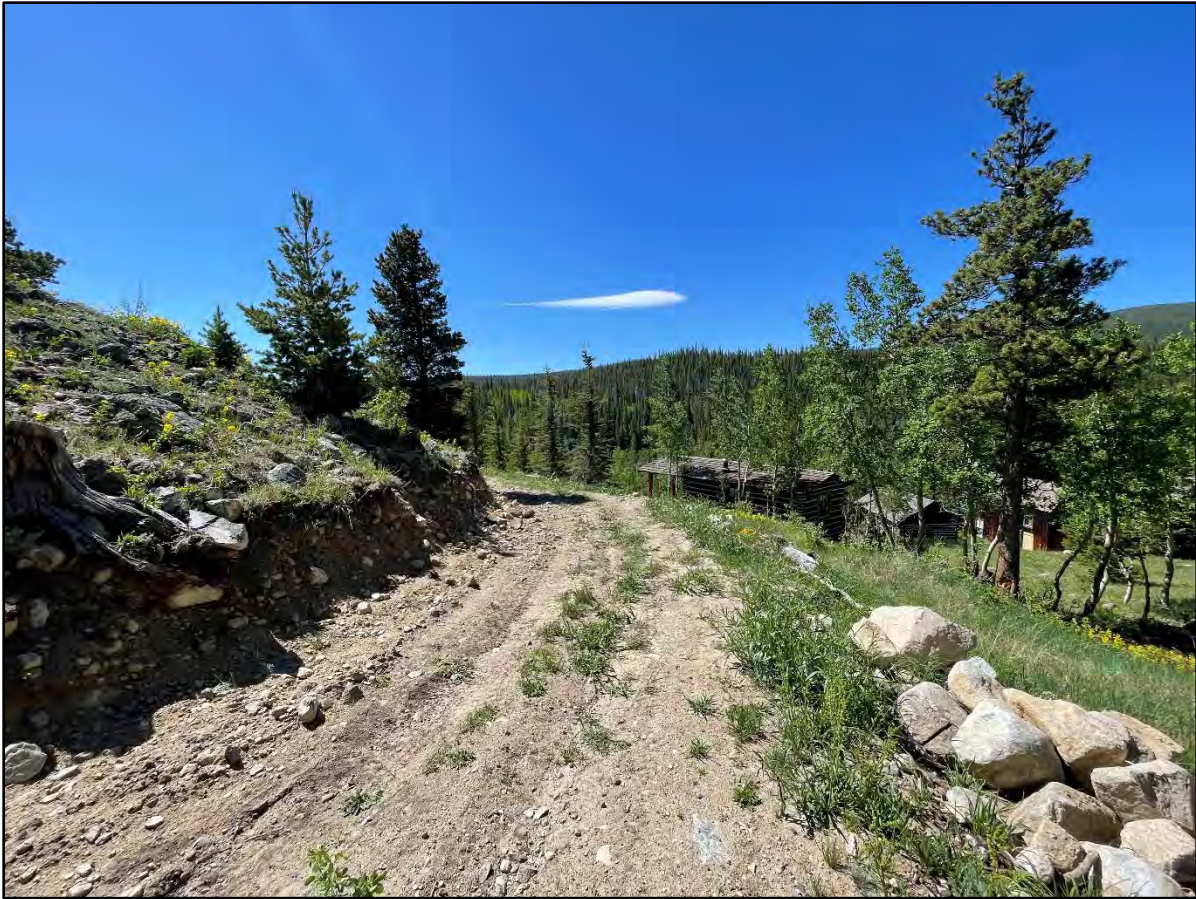
Photo 17. The partially improved road follows the alignment of an old forest road for most of its length. (6/17/24).
