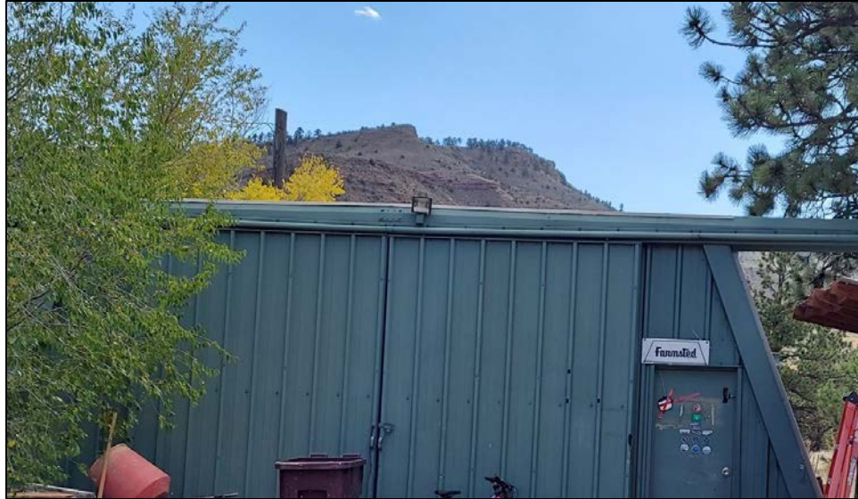
Figure 7: Photograph of existing structure, with non-compliant exterior light fixture.
